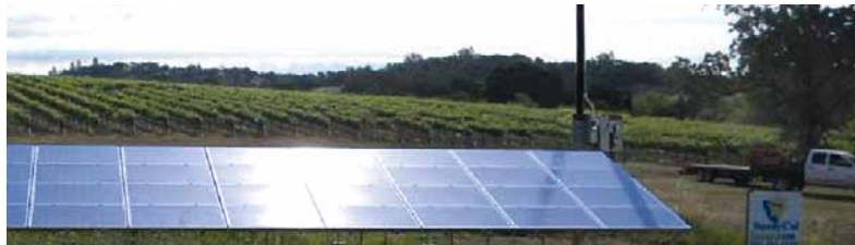
California’s salty coastal air is no problem for the C-Series modules.
