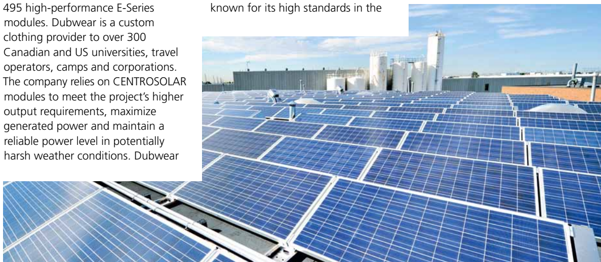
495 E-Series modules on the roof of Dubwear, in Canada.
